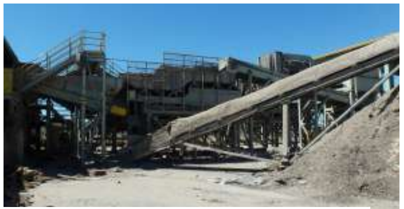
Figure 11. C&D Processing Line and Tipping Building
