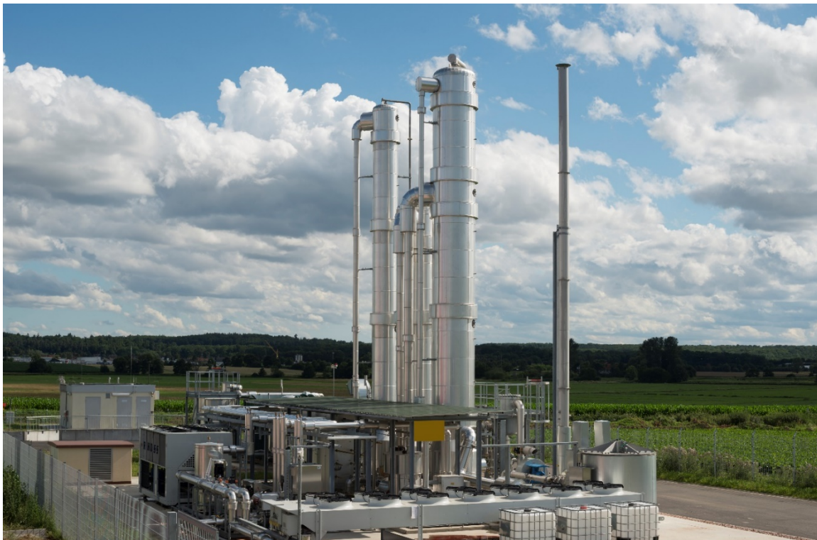
Figure 5-17. Representative Complementary and Programmatic Element – Biomass Facility Source: iStock
